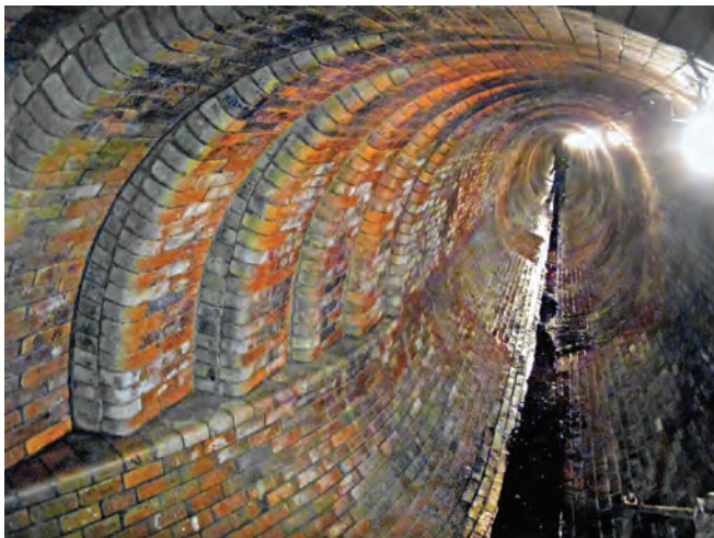
The overflow sewer that we traversed while viewing the underground settlement tanks
